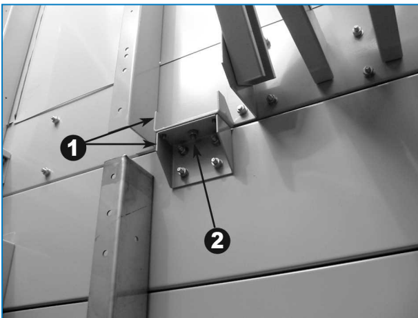
Plenum section installed on lower section
